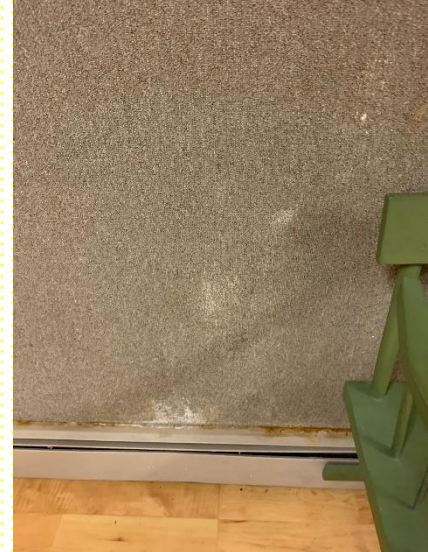
Electric Baseboard Heater Damage
